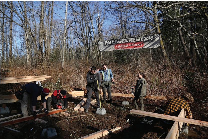
Figure 2. Volunteers help build the Kwekwecnewtxw, a traditional Coast Salish watch house, early Saturday morning on Burnaby Mountain. The watch house will be used to hold ceremonies and keep watch over Kinder Morgan pipeline construction.
