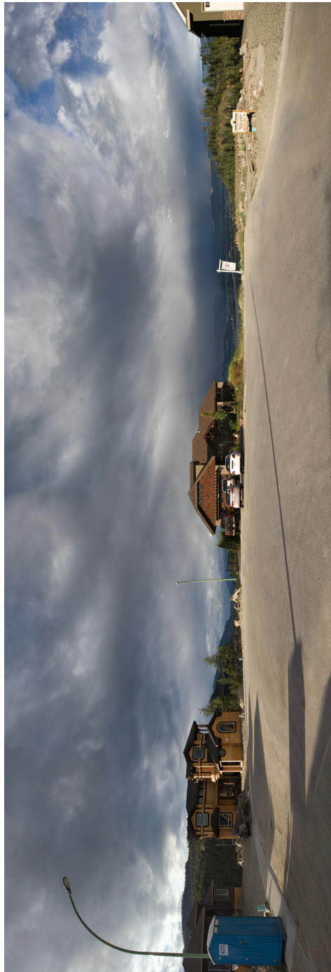
Top: Clearing land, future cul-de-sac, upper level, Panorama Peaks , 2003. Bottom: First completed house, upper level, cul-de-sac, Panorama Peaks , 2006.
