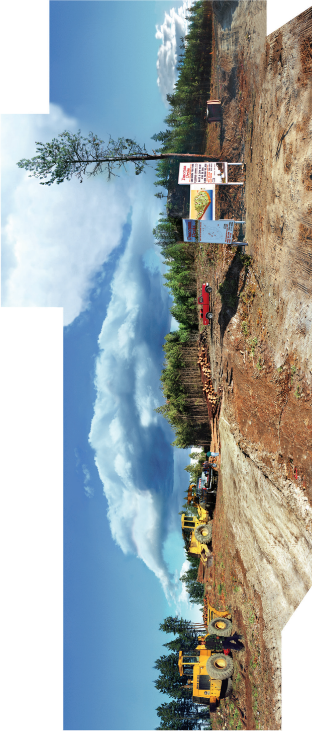
Clearing and preparing land. Future entrance to Panorama Peaks with remaining lone tree, 2003.
